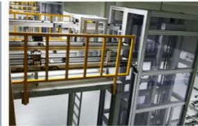
Air conveyor platform
